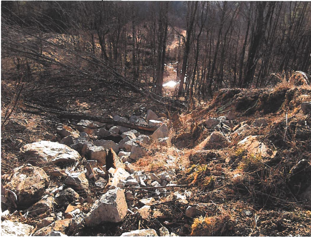
Photo of erosion before repairs:
